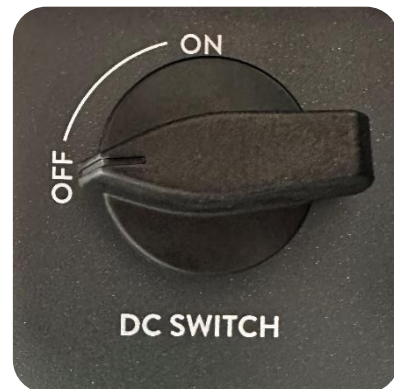
Figure 18: Deactivation of the photovoltaic direct current supply_1.1
