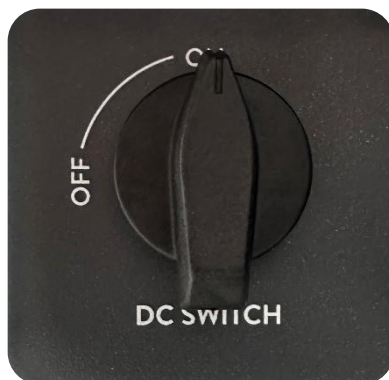
Figure 17: Deactivation of the photovoltaic direct current supply_1.1
