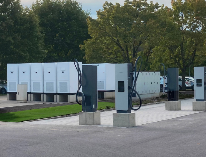
EV CHARGING PLAZA WITH CO-LOCATED G-MAX STORAGE
