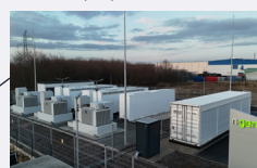
Vistula (PL) 9.4 MW / 18.8 MWh
